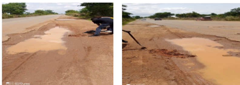
Fig 7: Some of the Many Scraped Shoulders (within 20-31km from origin)
