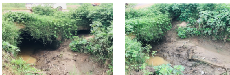
Fig 8 : Some of the few Blocked Culverts (located at about 2.1 and 13.5 km from origin respectively)
