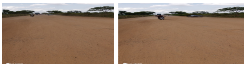
Fig 6: Some of the Many Areas with Erased Pavement Markings (within about 1-13km from origin)
