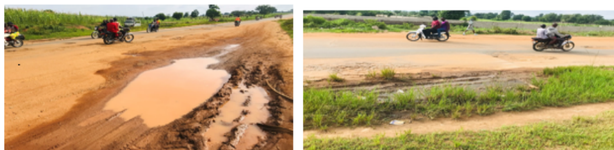
Fig 5: Some Effects of Lack of Drainages at about 31 km from the Origin
